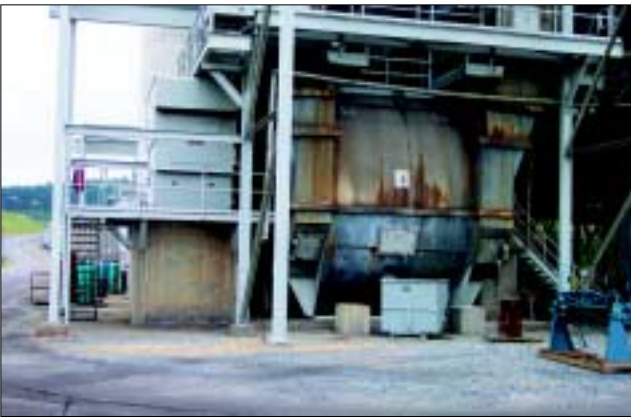
Figure 3. Fan housing and motor pedestal on embedded foundation.
