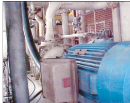
Figure 4. 350 hp centrifugal compressor.
