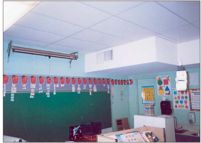
Figure 5. New supply air diffuser and duct enclosure.
