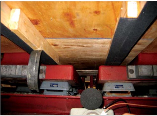
Figure 7. Plywood screen under genset.
