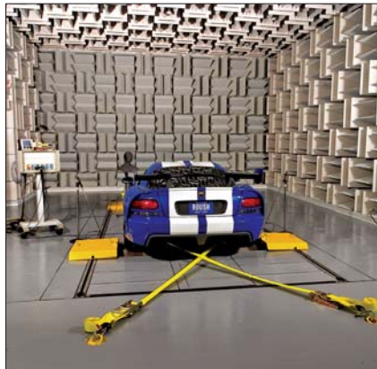
Figure 1. Roush's new hemi-anechoic chamber was designed and installed by Eckel Industries and provides a controlled acoustic environment for NVH services.
