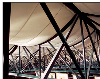
Figure 3. Close-up view of typical installation.
