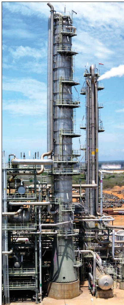
Figure 1. High-displacement, low-frequency vibration developed atop a large process column.
