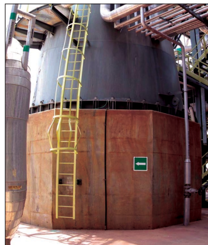
Figure 3. Massive foundation of the column was included in the 3-D finite-element model.
