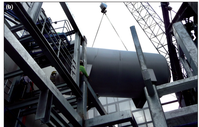
Figure 5. Various facility noise mitigation measures: (a) lube oil cooler acoustical barrier; (b) steam bypass silencer.
