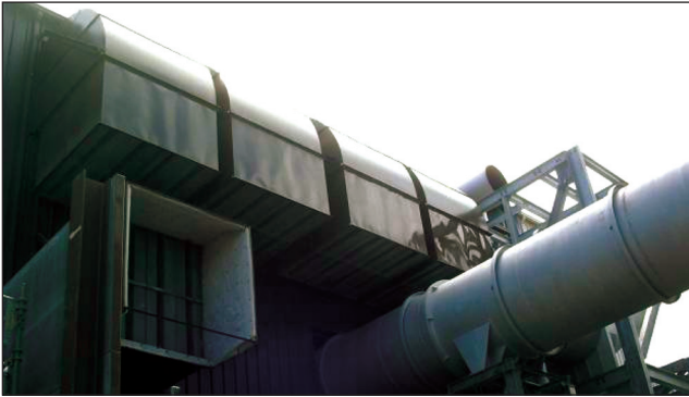
Figure 3. STG building ventilation acoustical hoods.
