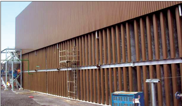
Figure 4. Air-cooled condenser inlet acoustical baffles.
