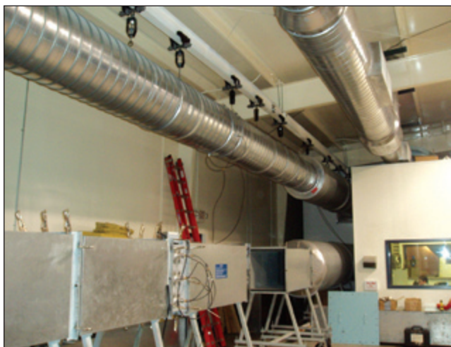
Figure 4. Test duct showing lagged rectangular ductwork prior to test specimen with duct downstream encased inside a spiral round duct.
