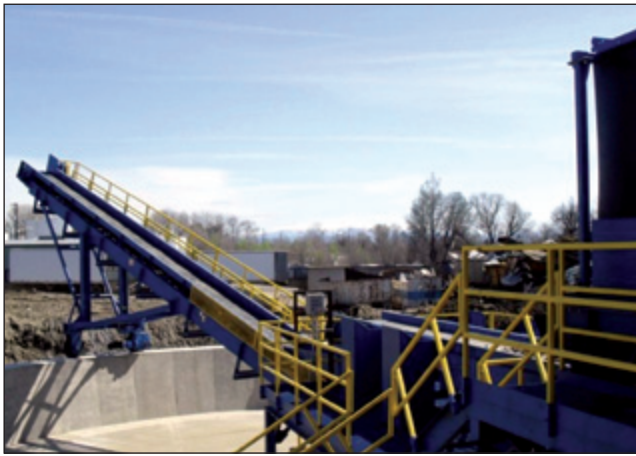
Figure 2. Shredder system conveyor.
