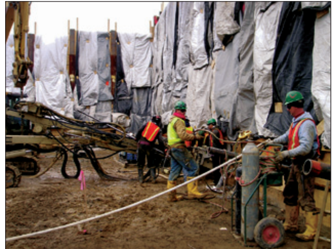
Noise-control curtains being used to reduce noise emissions from a rock-drilling operation to the surrounding community.
