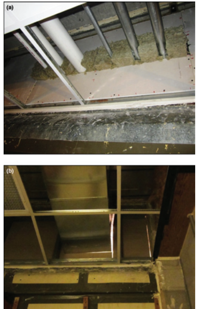
Figure 4. A quick installation technique was used for some of the drywall barriers: (a) large openings were left around the penetrating elements so simple rectangular pieces of drywall could be used; those openings were stuffed with pieces of stone wool insulation; (b) large gaps between pieces of drywall and around the penetrating elements were not caulked or taped; light shining through the gaps from the opposite side of the barrier show their size and extent.
