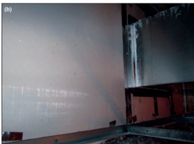
Figure 5. A sealed installation technique was used for some of the drywall barriers: (a) drywall was cut closely around the penetrating elements and caulked; (b) joints, screw heads and penetrations were sealed with metal tape.
