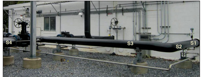
Figure 8. Suction piping vibration data points.
