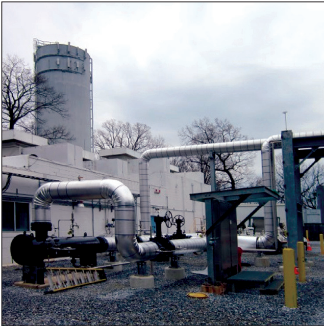
Figure 17. Exposed yard piping with acoustic insulation installed.
