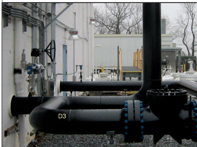
Figure 13. Section of discharge piping where standing wave was suspected.
