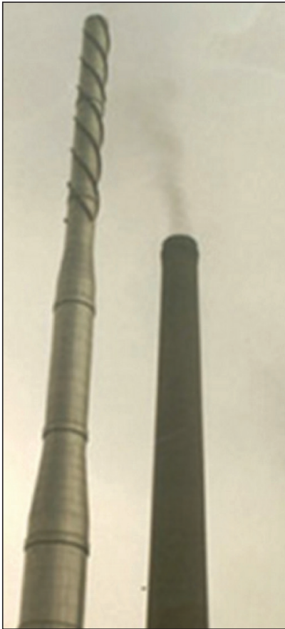
Figure 8. Helical strakes across part of chimney (left) control vortex excitations.
